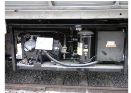
2 New AC Units
